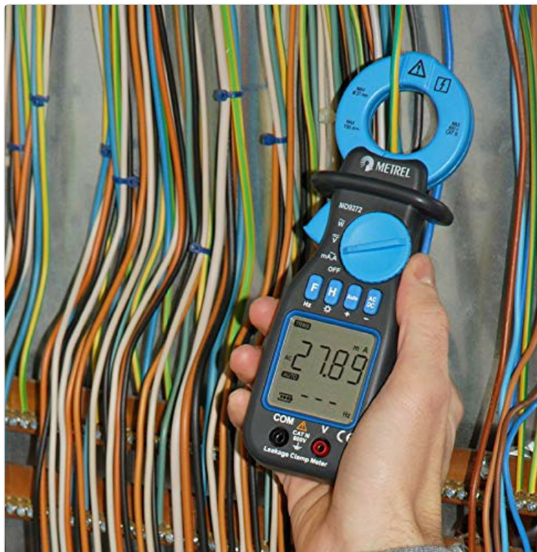
Figure 1: The Metrel MD 9272 Leakage Clamp Meter in use. This image shows the device being held by a hand, with its clamp jaw around a bundle of electrical wires. The display shows a reading of 27.89 mA, indicating current measurement. The
