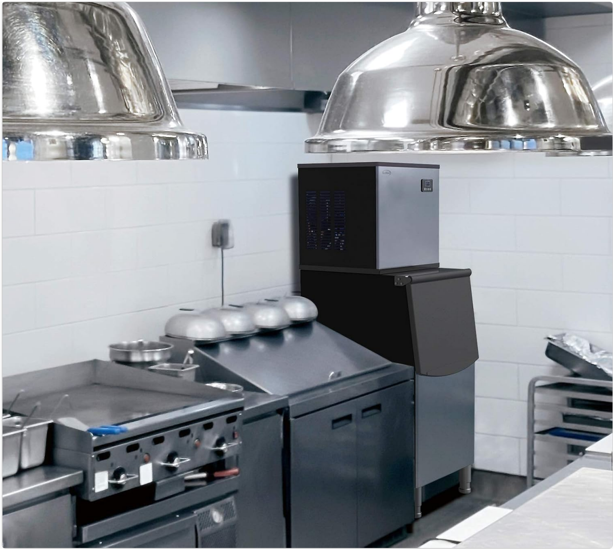
Image 2: The ice maker installed in a commercial kitchen, demonstrating appropriate placement.
