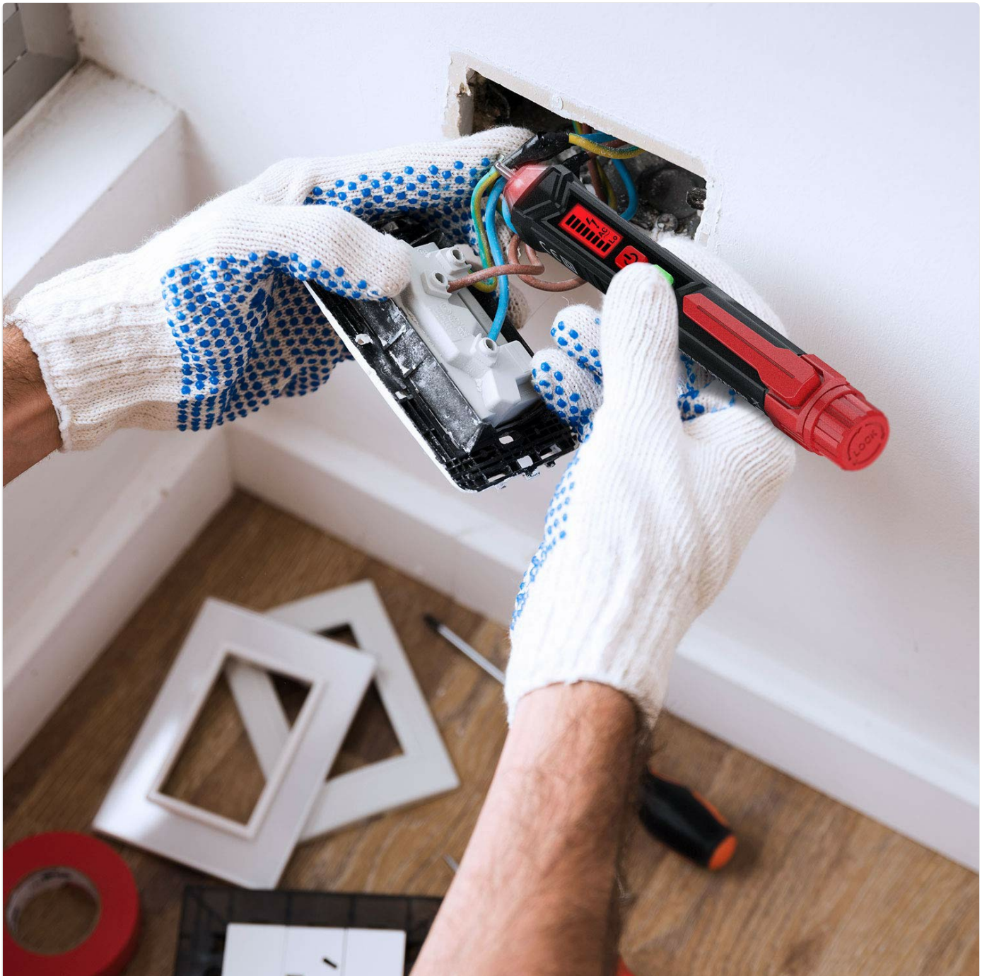
Figure 3.3: The NCV tester in use, checking for voltage in an electrical box.
