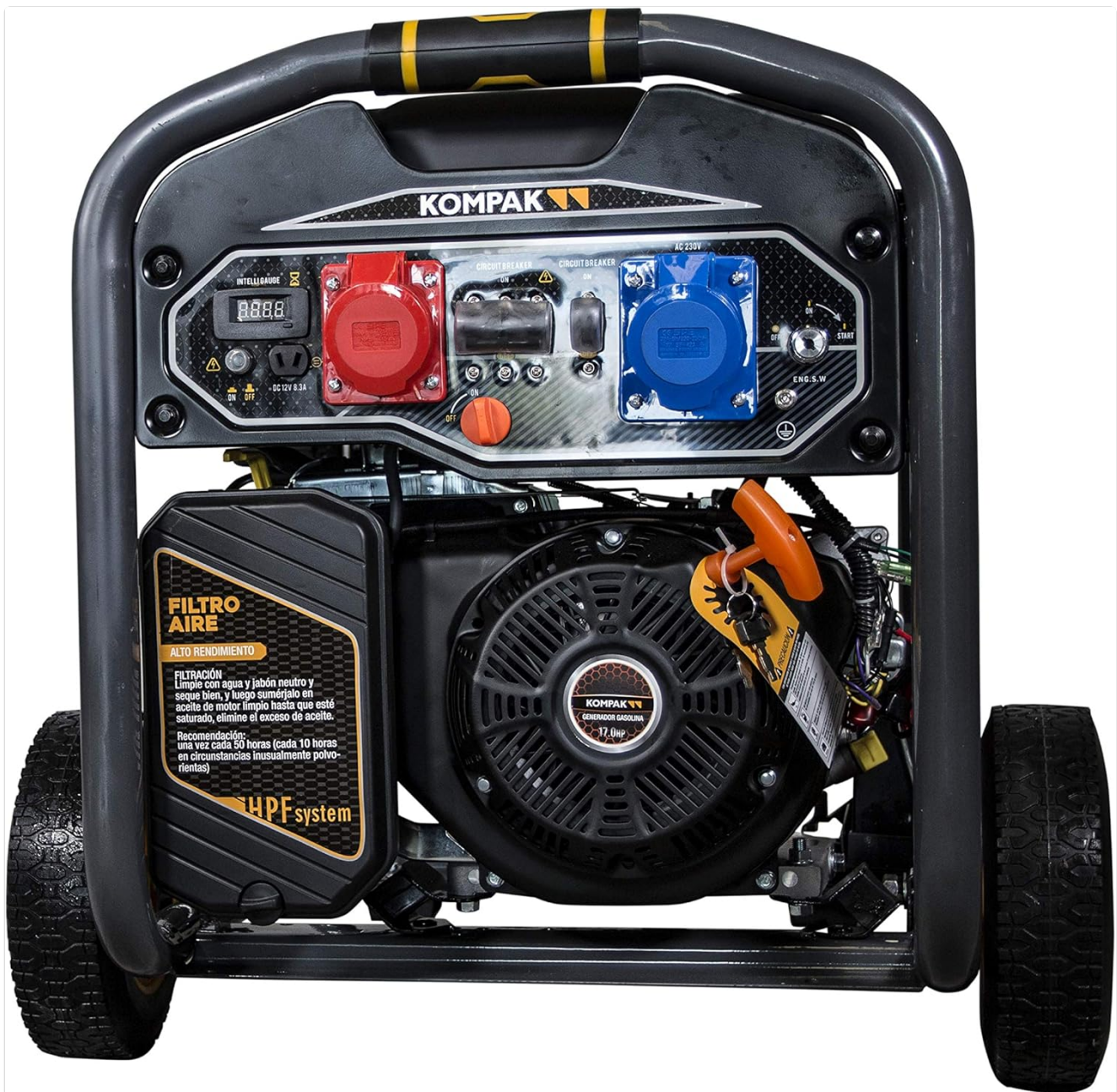
Figure 5.1: Close-up of the generator's control panel, showing the various switches, outlets, and indicators for operation.
