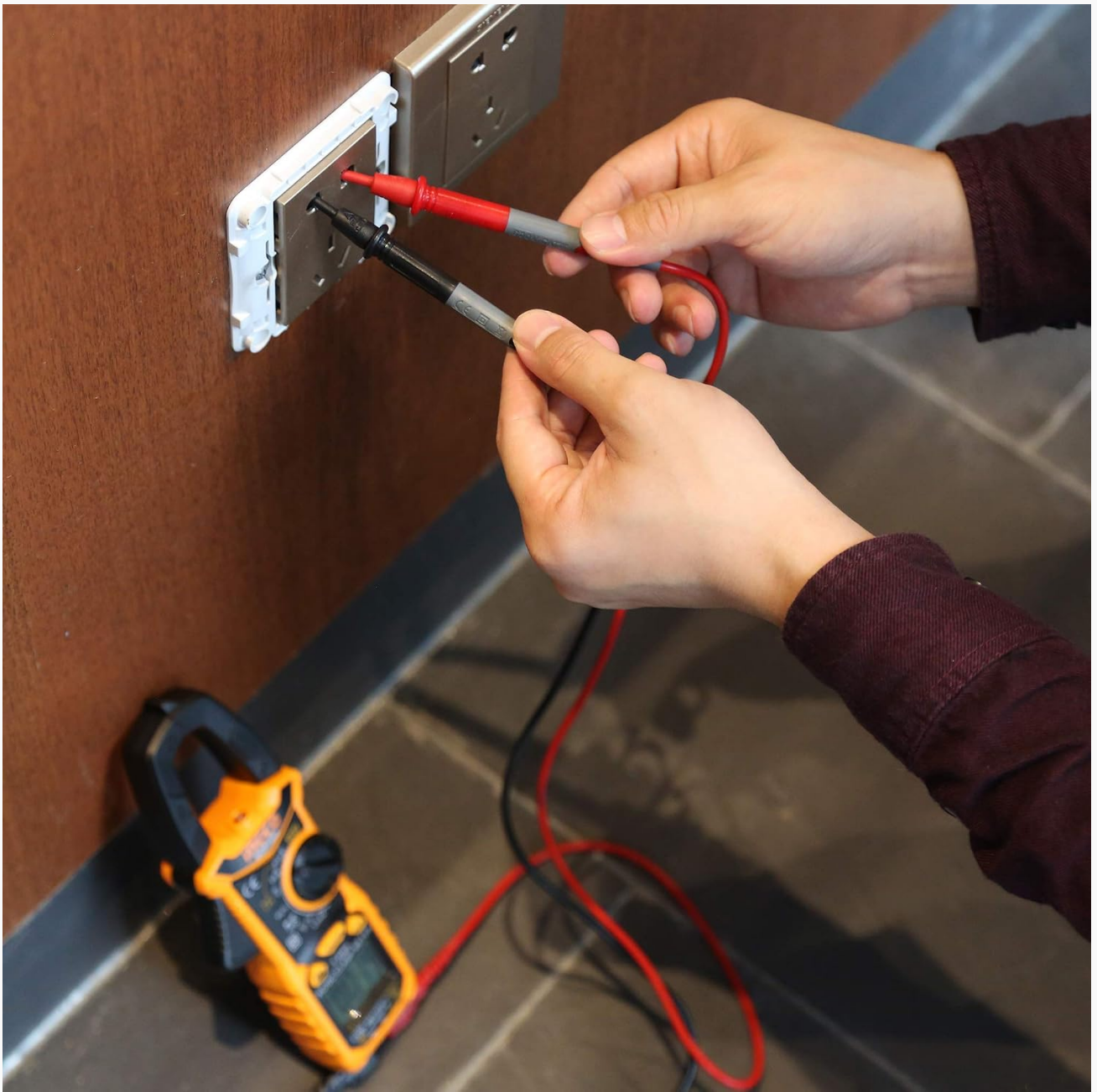
Image: A user holding the red and black test leads from the DCM6005 to measure AC voltage at a wall outlet, with the clamp meter resting on the floor nearby.
