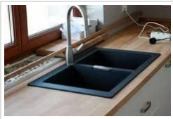
Image: Franke S2D 620 sink installed in a kitchen countertop, demonstrating a typical flush-mounted setup with a faucet.
