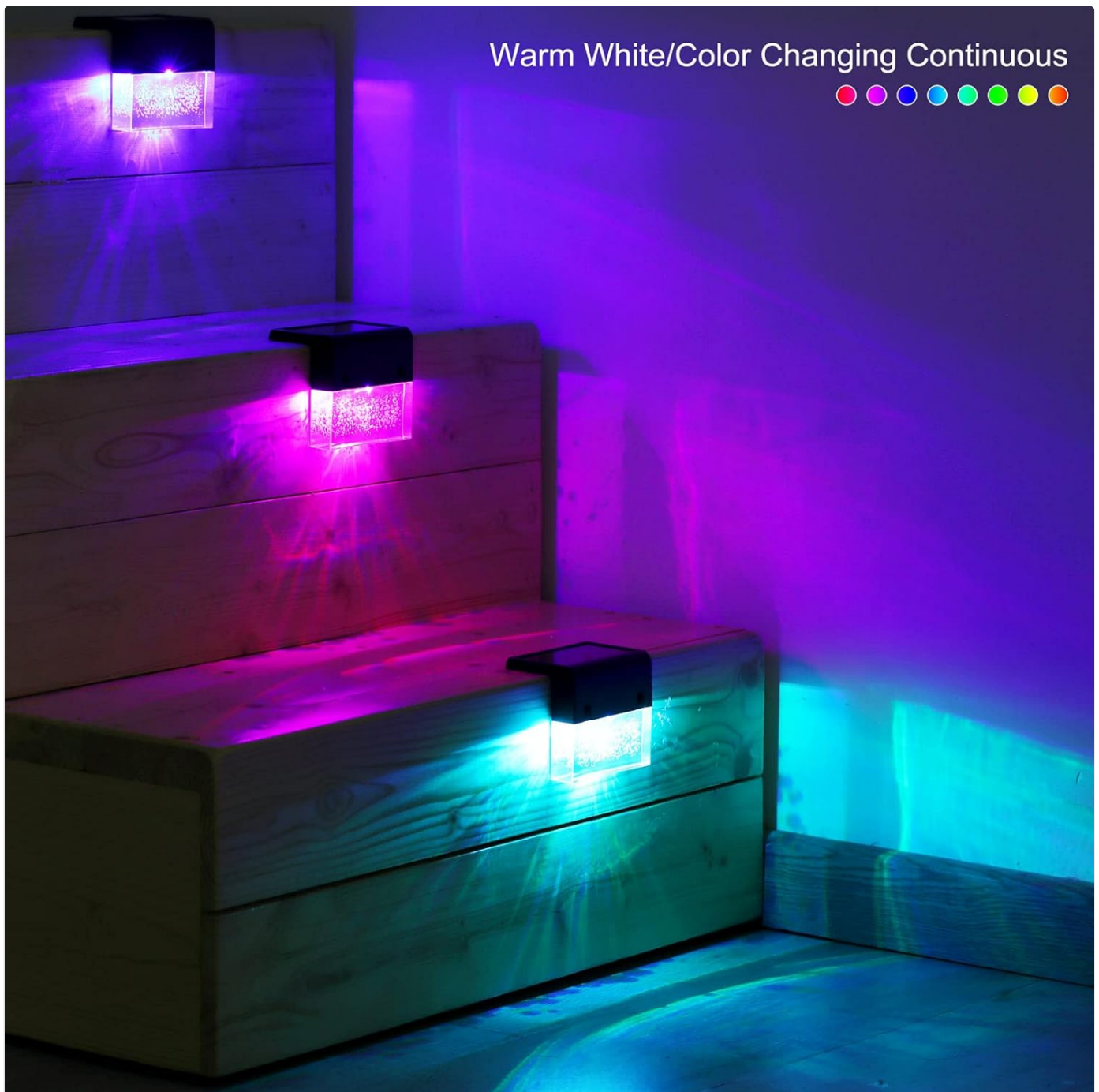
Image: Solar deck lights installed on wooden steps, showcasing both warm white and continuous color-changing illumination.
