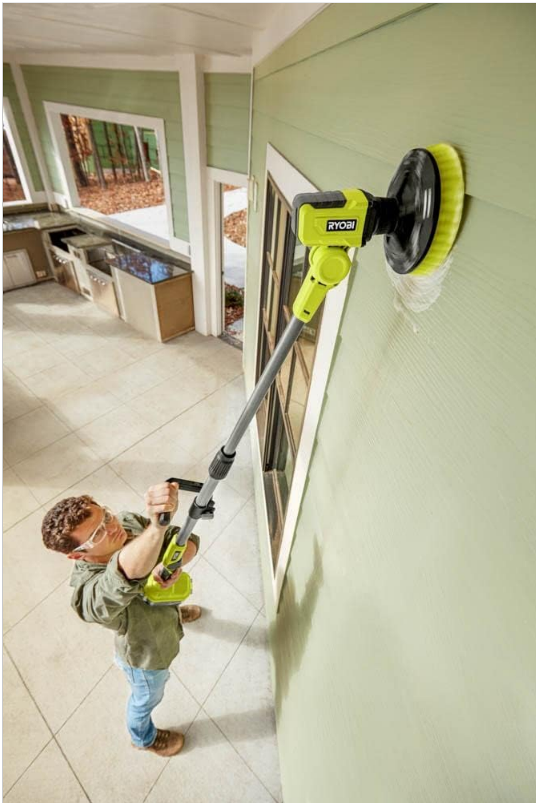
Figure 3: Demonstrating the extended reach of the power scrubber for cleaning high surfaces.
