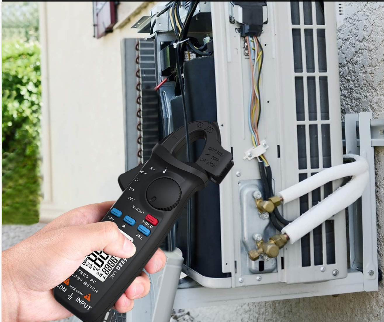
Image 5.2.1: The clamp meter is shown in use, measuring the AC current flowing through a single conductor of an outdoor air conditioning unit.
