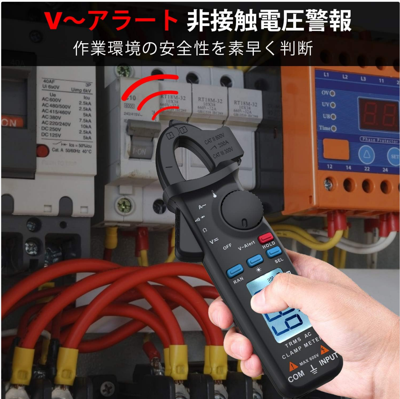
Image 5.7.1: The clamp meter is used to detect non-contact voltage near a circuit breaker panel, indicating the presence of live AC voltage.
