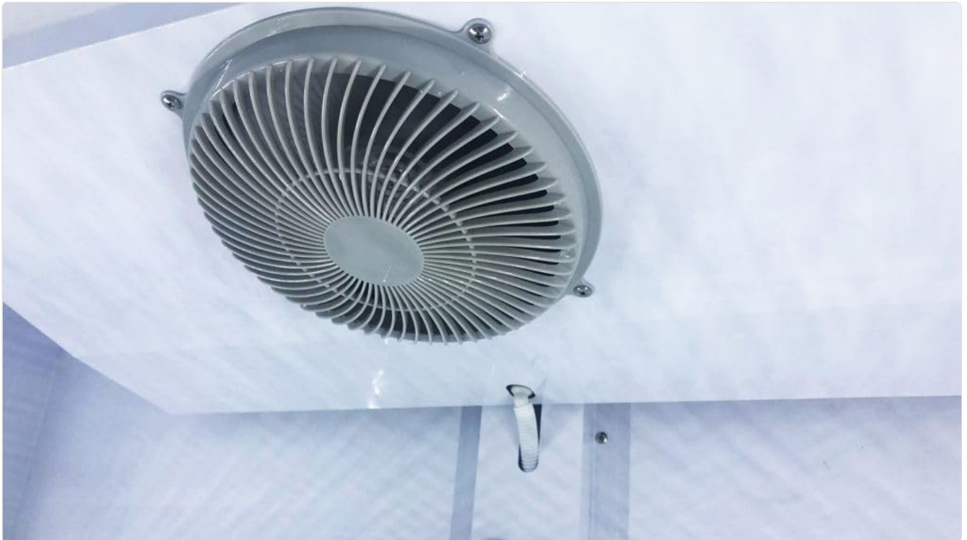
Figure 6: Close-up view of the interior ceiling, showing the two circulation fans.
