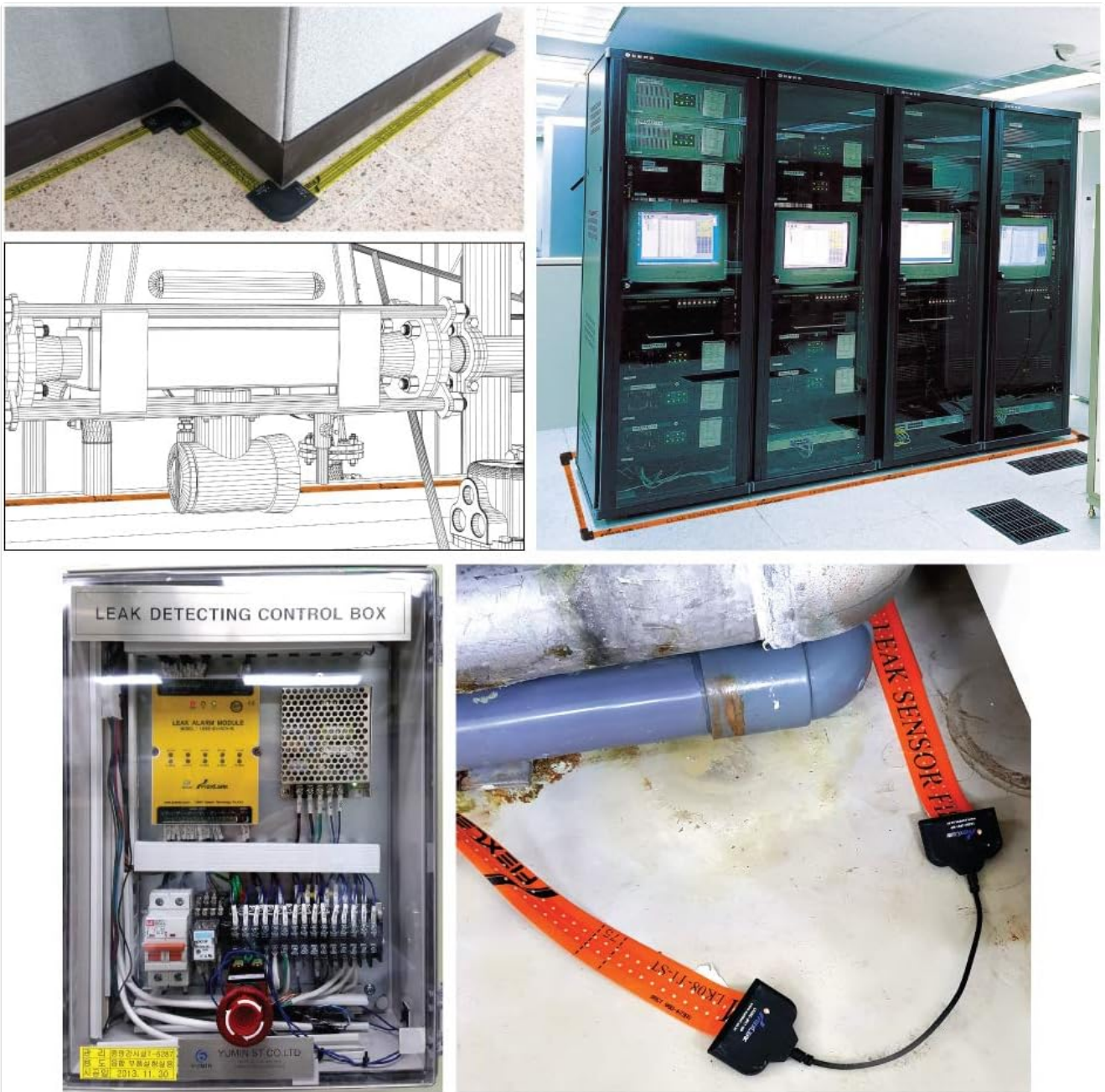
Figure 3.3: Examples of the FLEXLEAK system installed in various environments, including server rooms, near pipes, and along walls.
