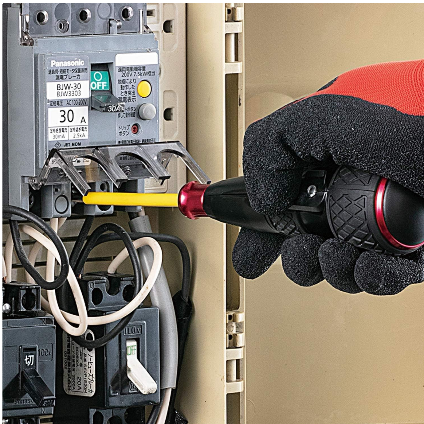
Figure 3: The electric driver being used for electrical panel work, demonstrating its application in tight spaces.
