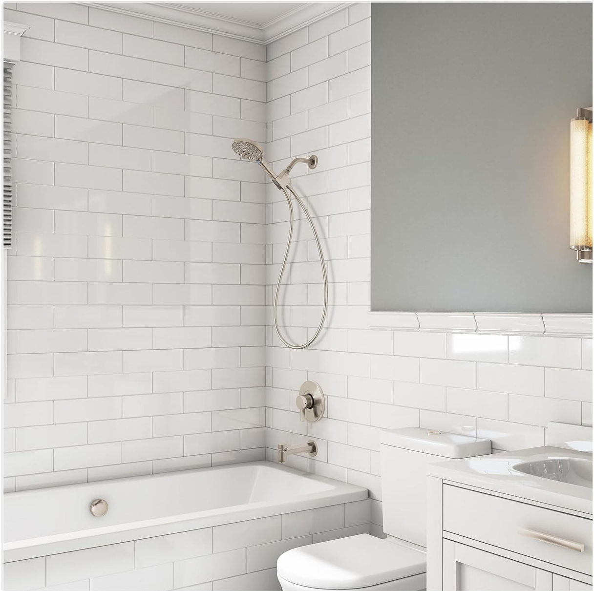
Figure 2: The complete hansgrohe shower set installed, showing the handshower in its mount and the flexible hose.
