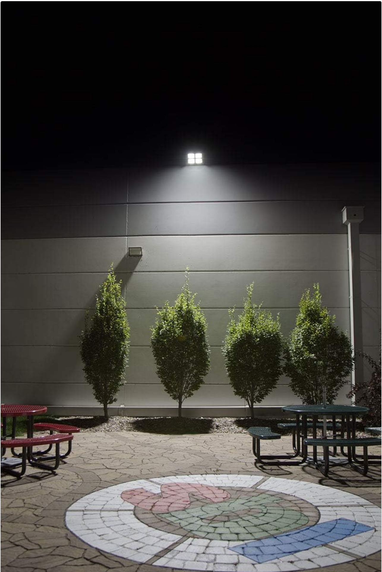
Figure 5: Example of the flood light in operation, illuminating an outdoor area.
