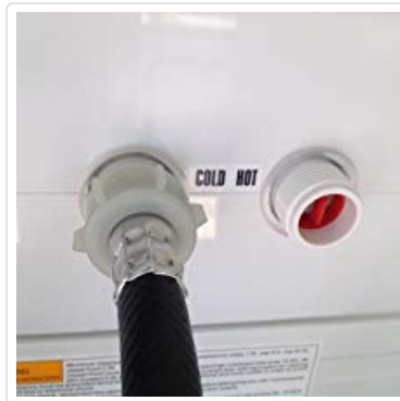
Image: Close-up of the cold water inlet on the back of the washer, showing a hose connected and the hot inlet plugged.
