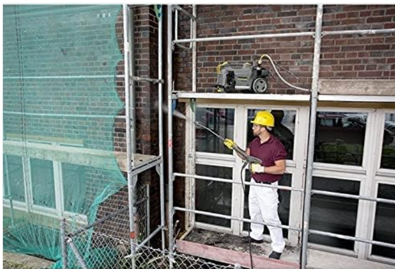
Figure 4: Demonstrating the effective cleaning power of the Kärcher HD 6/13 C on a graffiti-covered wall.
