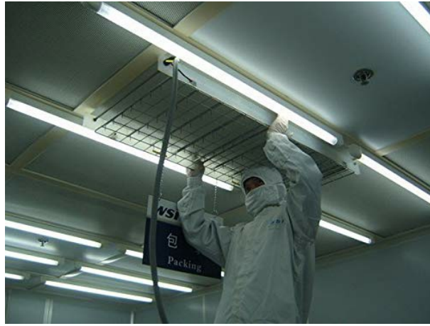
Figure 5.1: Example of Anti-static Ionizer Net installation. A technician in protective gear is shown installing the ionizer net into a ceiling grid, demonstrating typical placement in a controlled environment.
