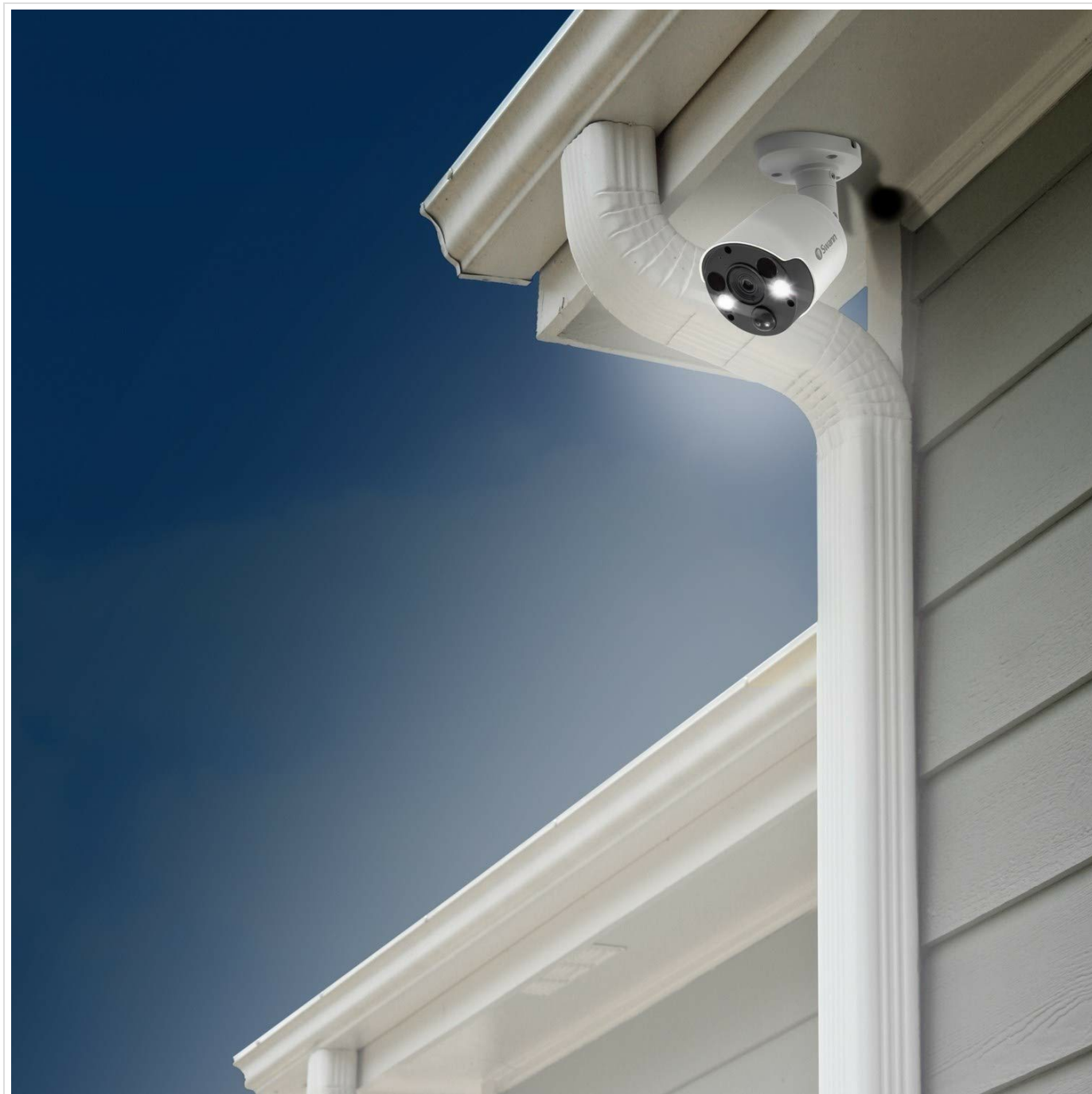
Image: The Swann PRO-5MPMSFB camera installed on the exterior wall of a house, positioned near a downspout, with its spotlights active and casting light downwards.
