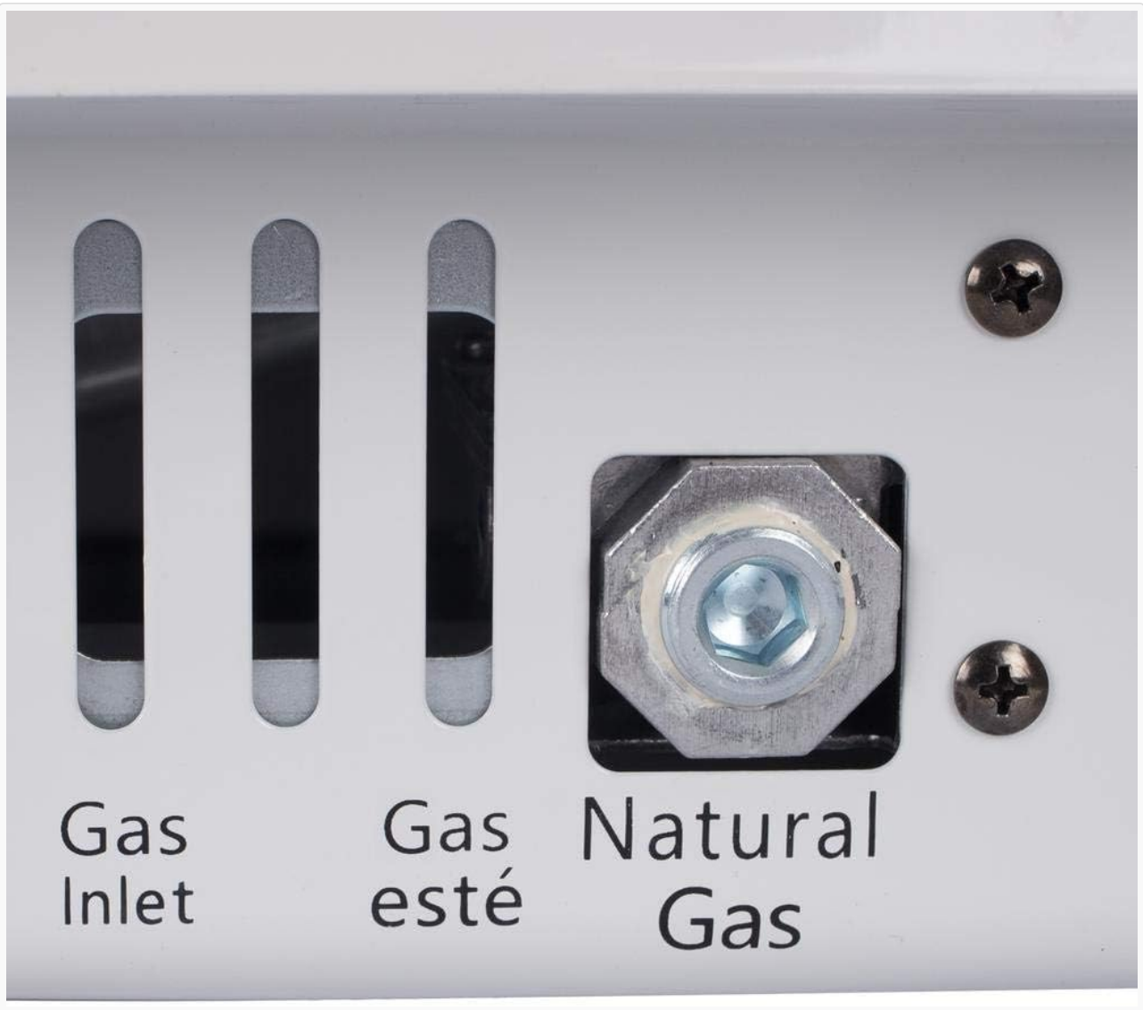
Natural gas inlet connection point.
