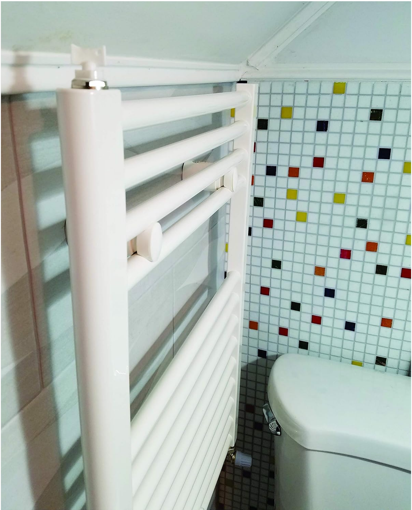
Image 1.2: The Cordivari Lisa 22 Towel Warmer installed in a bathroom, demonstrating its integration into a typical bathroom setting next to a toilet and tiled wall.
