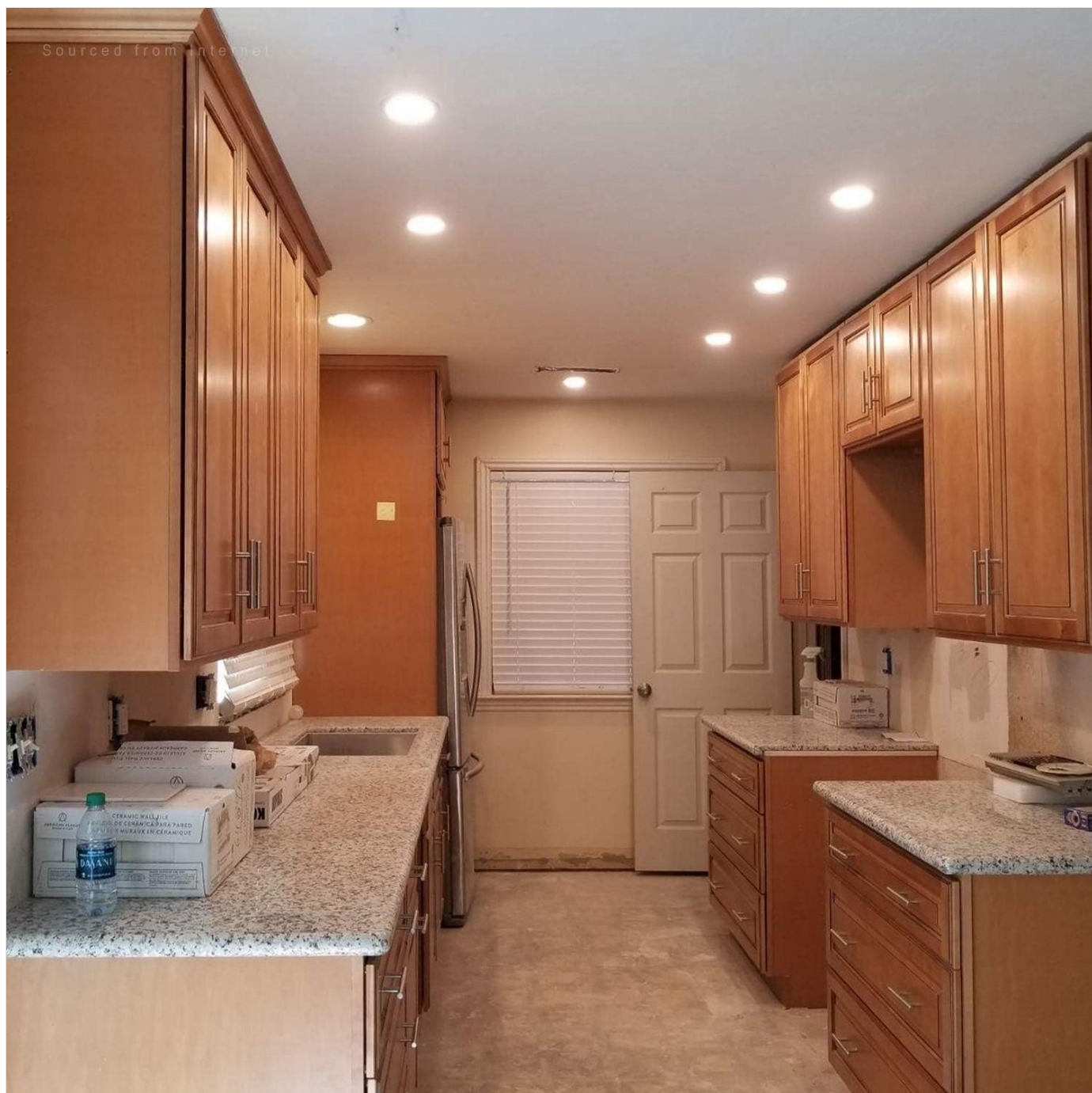
Image 6.4: Example of installed recessed lighting in a kitchen environment.
