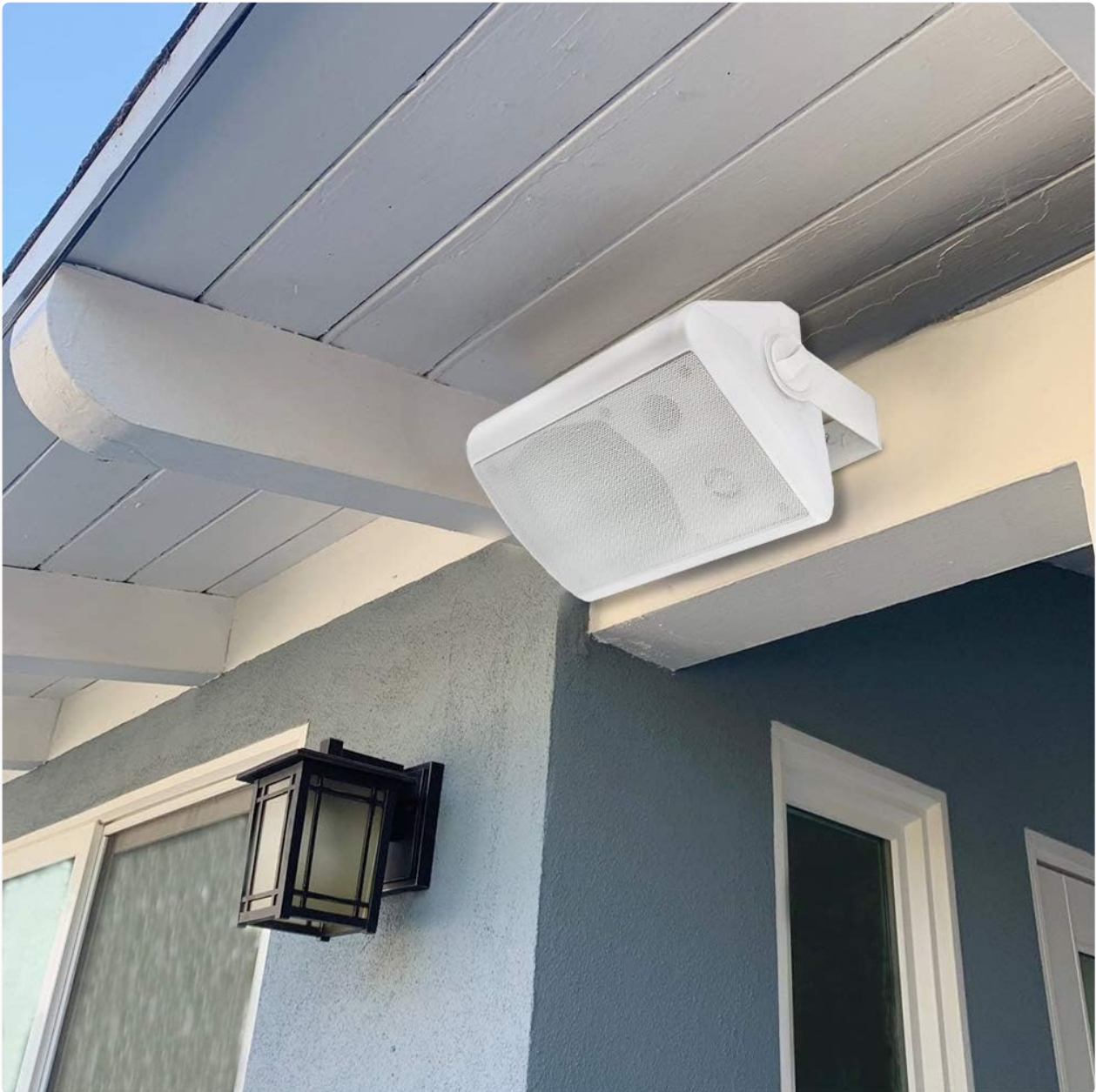
Image: An installed Herdio outdoor speaker mounted under an eave, demonstrating a typical installation scenario.
