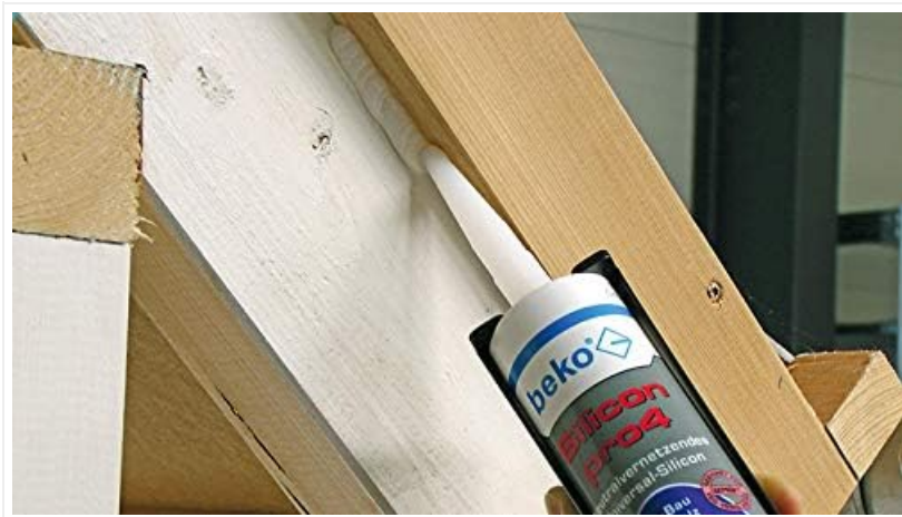
Image 4.2: Sealing a wooden frame with Beko Silicon pro4, highlighting its use in carpentry and window installations.
