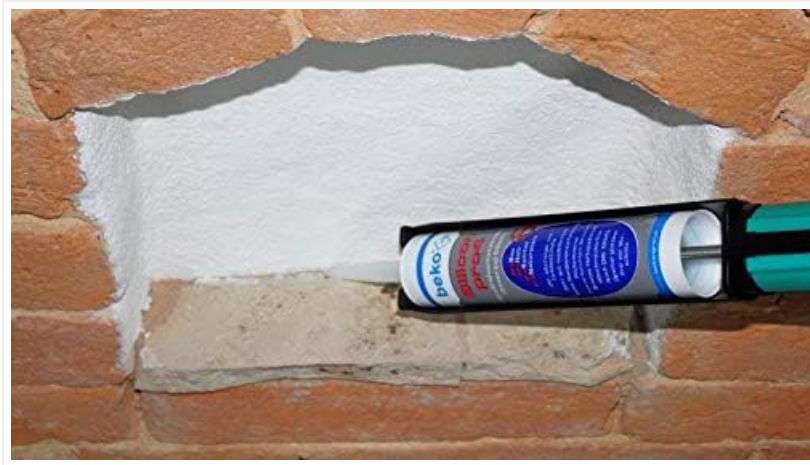
Image 4.1: Application of Beko Silicon pro4 into a joint on a brick wall, demonstrating proper technique.
