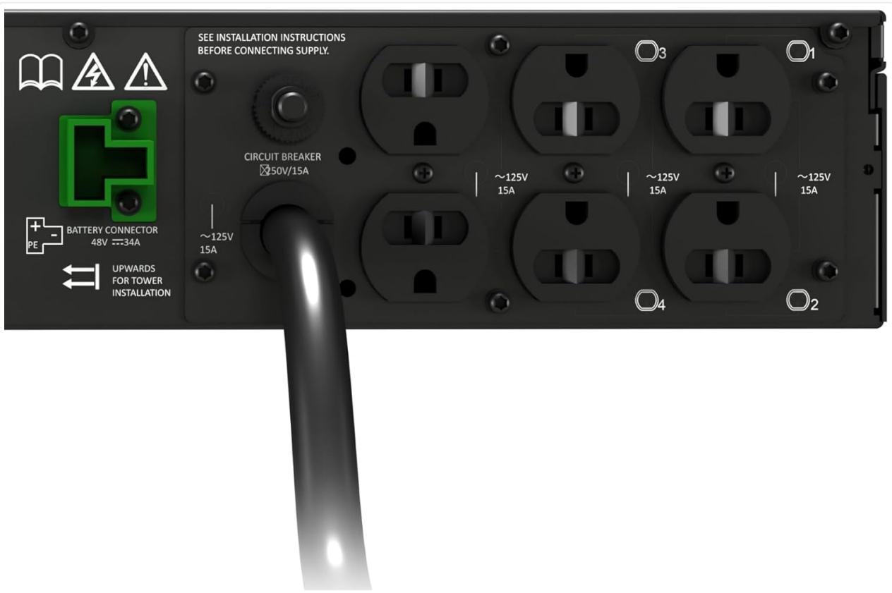
Figure 3: Detailed view of the UPS output receptacles.
