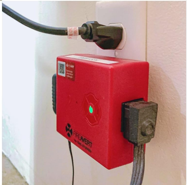
Figure 6: FireAvert unit installed behind the stove, connecting the stove to power.
