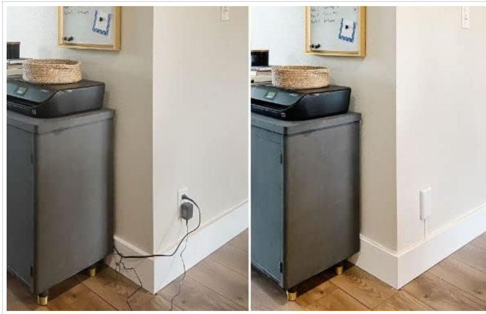
Image 5.4: Before and after installation behind a cabinet, demonstrating effective cord concealment.
