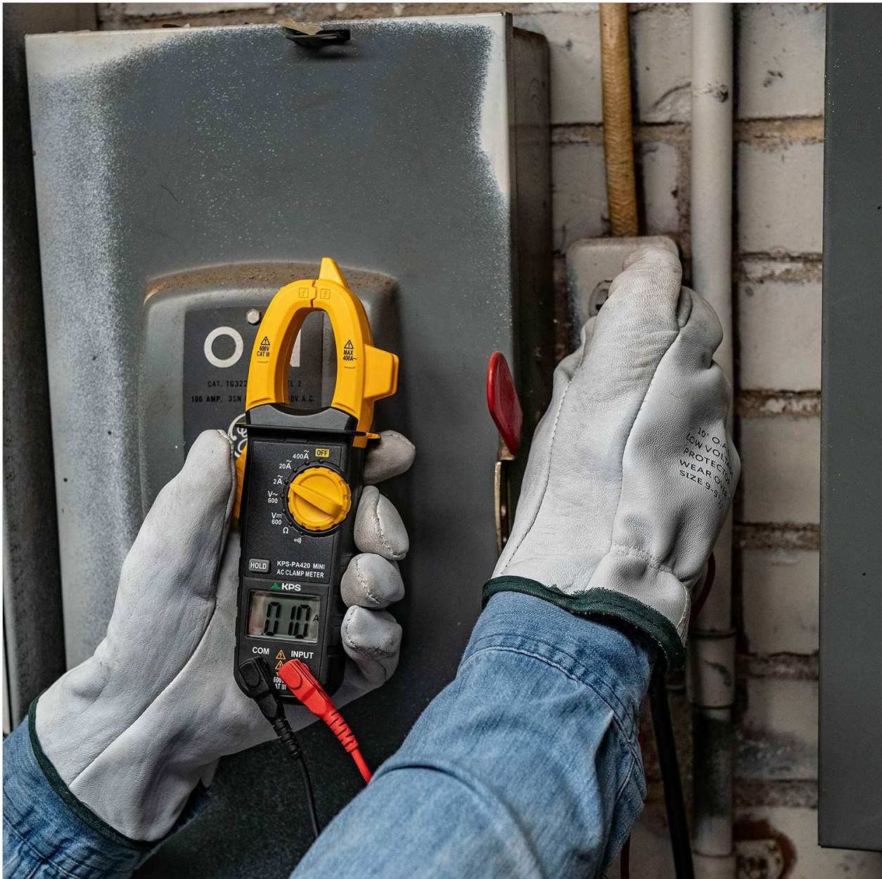
Image: A KPS-PA420 Mini Digital Clamp Meter with its test leads connected to an electrical panel, demonstrating voltage measurement.
