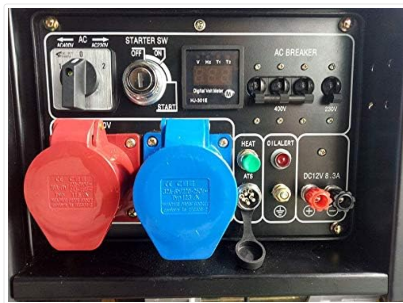
Figure 3.3: Detail of the VTS switch, indicating positions for AC 400V, Off (0), and AC 230V.
