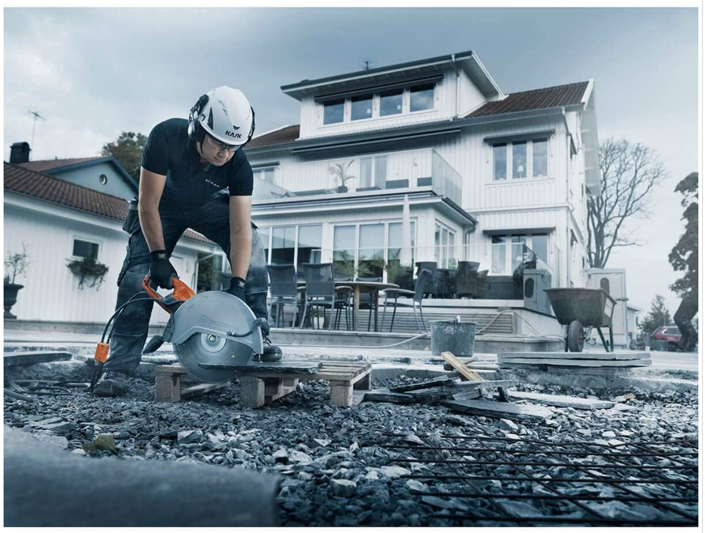
Image 2: An operator wearing safety gear, demonstrating the use of the Husqvarna K4000 Power Cutter Saw for cutting concrete outdoors.
