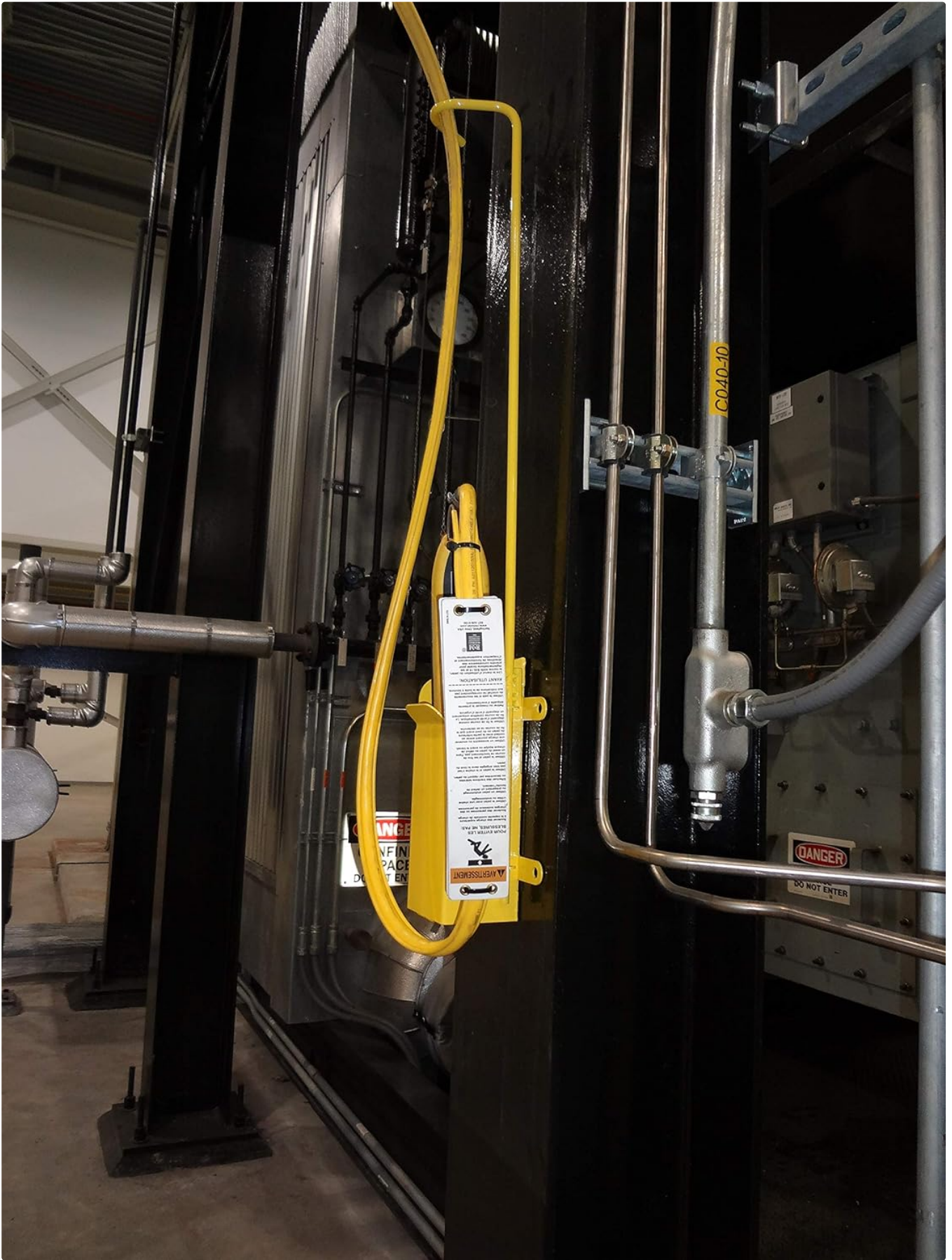
Figure 3.2.2: Another view of the S-PCM in an industrial environment, showing the pendant securely held within the box and the cable neatly routed through the support arm, enhancing safety and organization.
