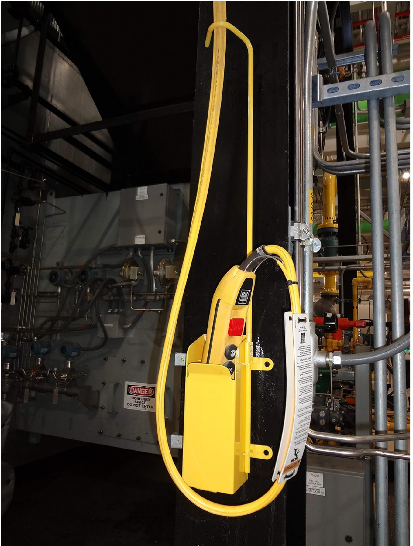
Figure 3.2.1: S-PCM installed on a structural beam, demonstrating how a crane pendant is stored and its cable is managed. The cable is looped through the support arm, keeping it organized and off the floor.
