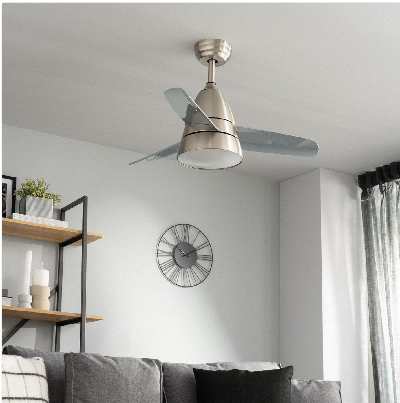
Figure 6: The ceiling fan installed and operating in a modern living room setting. This image shows the fan in its intended environment, demonstrating its aesthetic integration.
