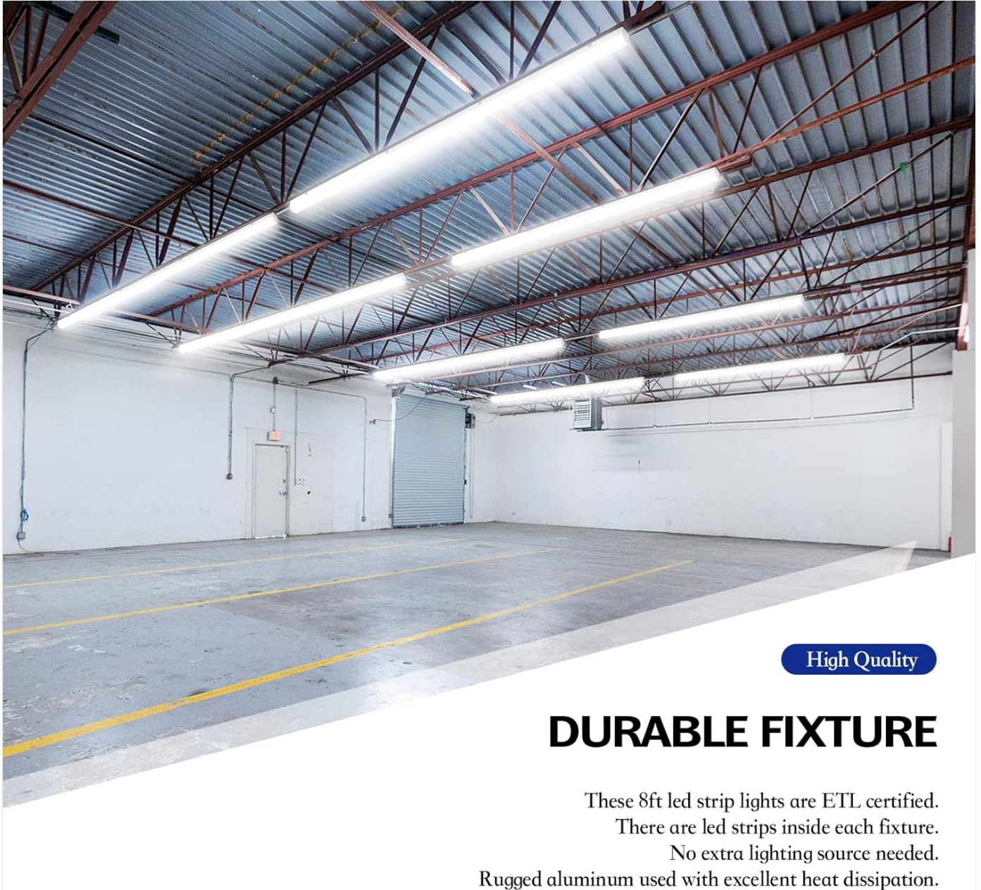
Image 6.1: ANTLUX lights providing illumination in a large space.
