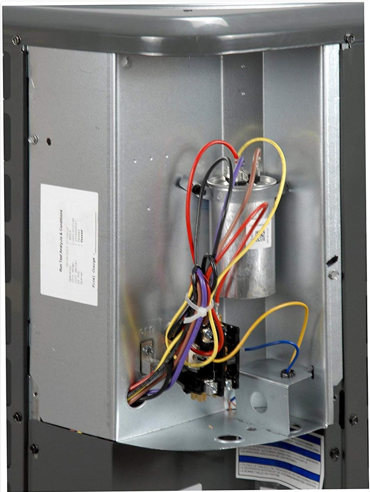
Figure 3: Close-up of the electrical wiring and capacitor, critical components for unit operation.
