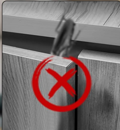
Cabinet doors not closing properly
