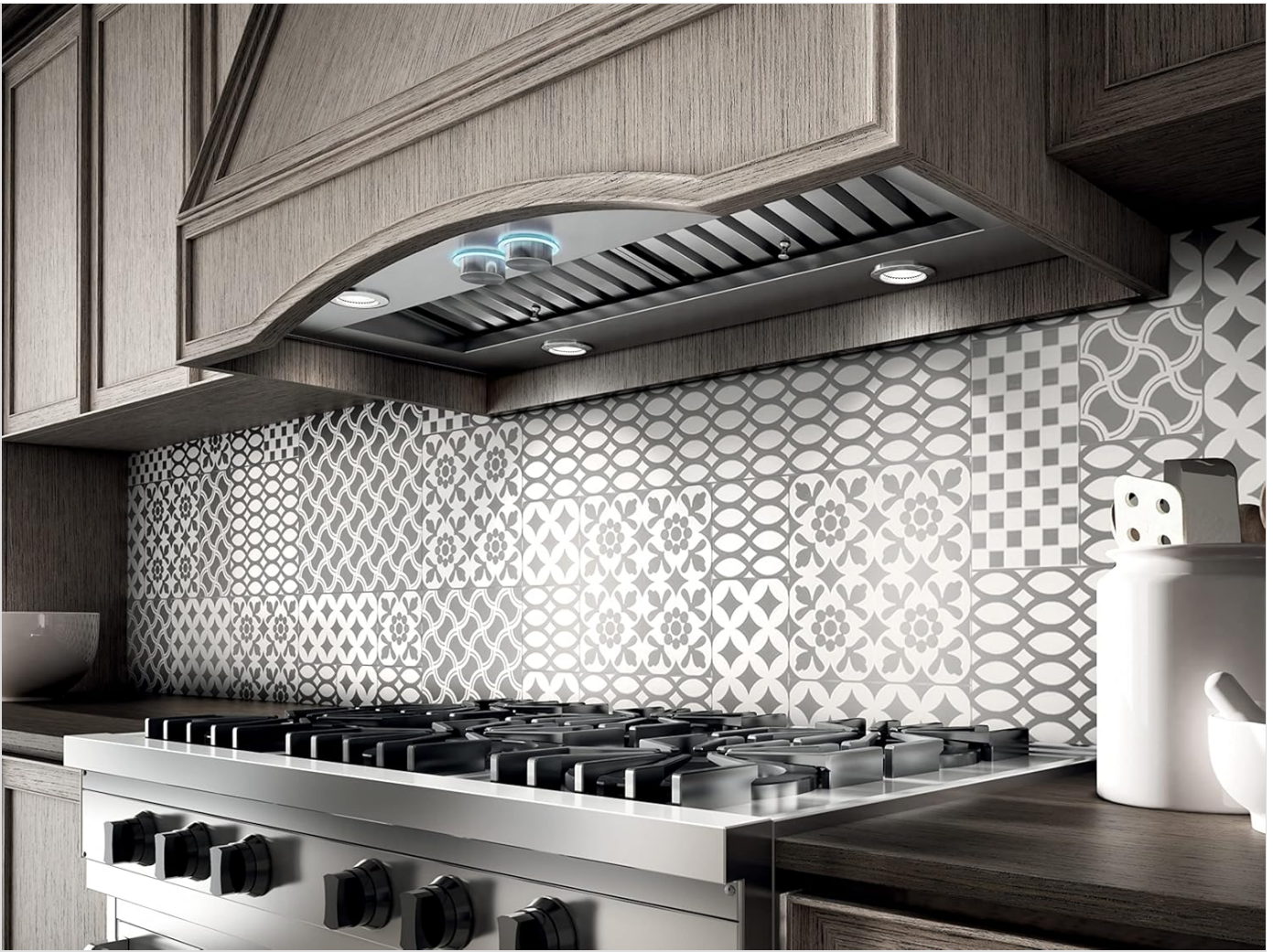
Another view of the Elica range hood installed above a cooktop, highlighting its discreet yet powerful presence.
