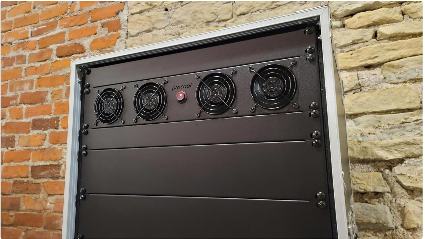
Figure 5.1: The PROCOOL T2280 unit installed within a server rack, demonstrating its 2U form factor and integration.
