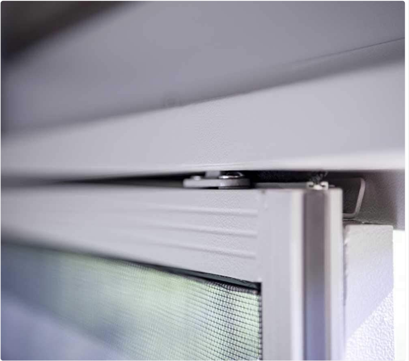
Figure 3.2: View of the top track system for the sliding doors.
