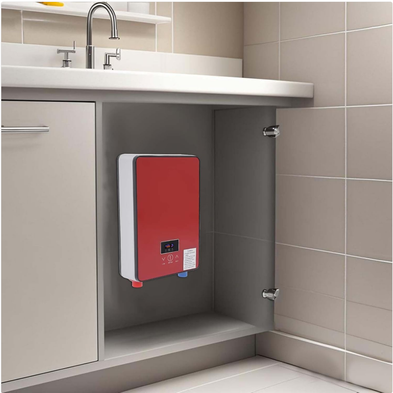
Image: The red tankless water heater unit discreetly installed inside a cabinet under a bathroom sink, demonstrating a common installation scenario.
