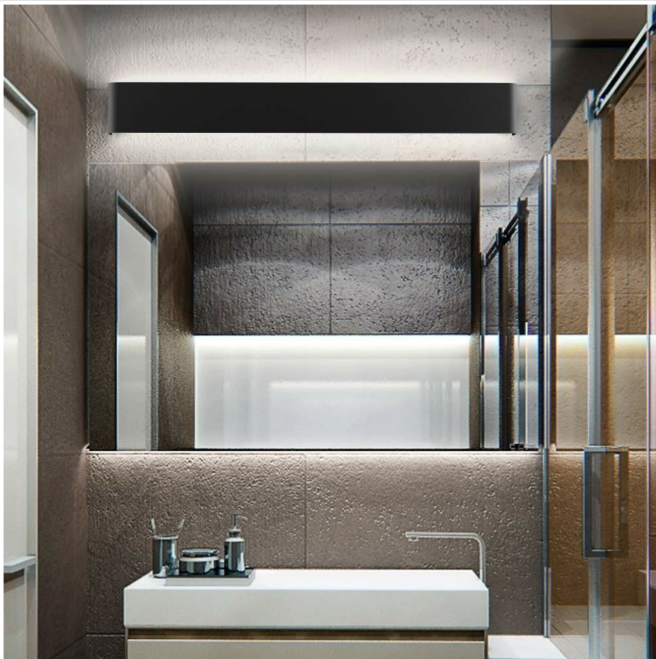
Image: Light fixture installed in a bathroom.
