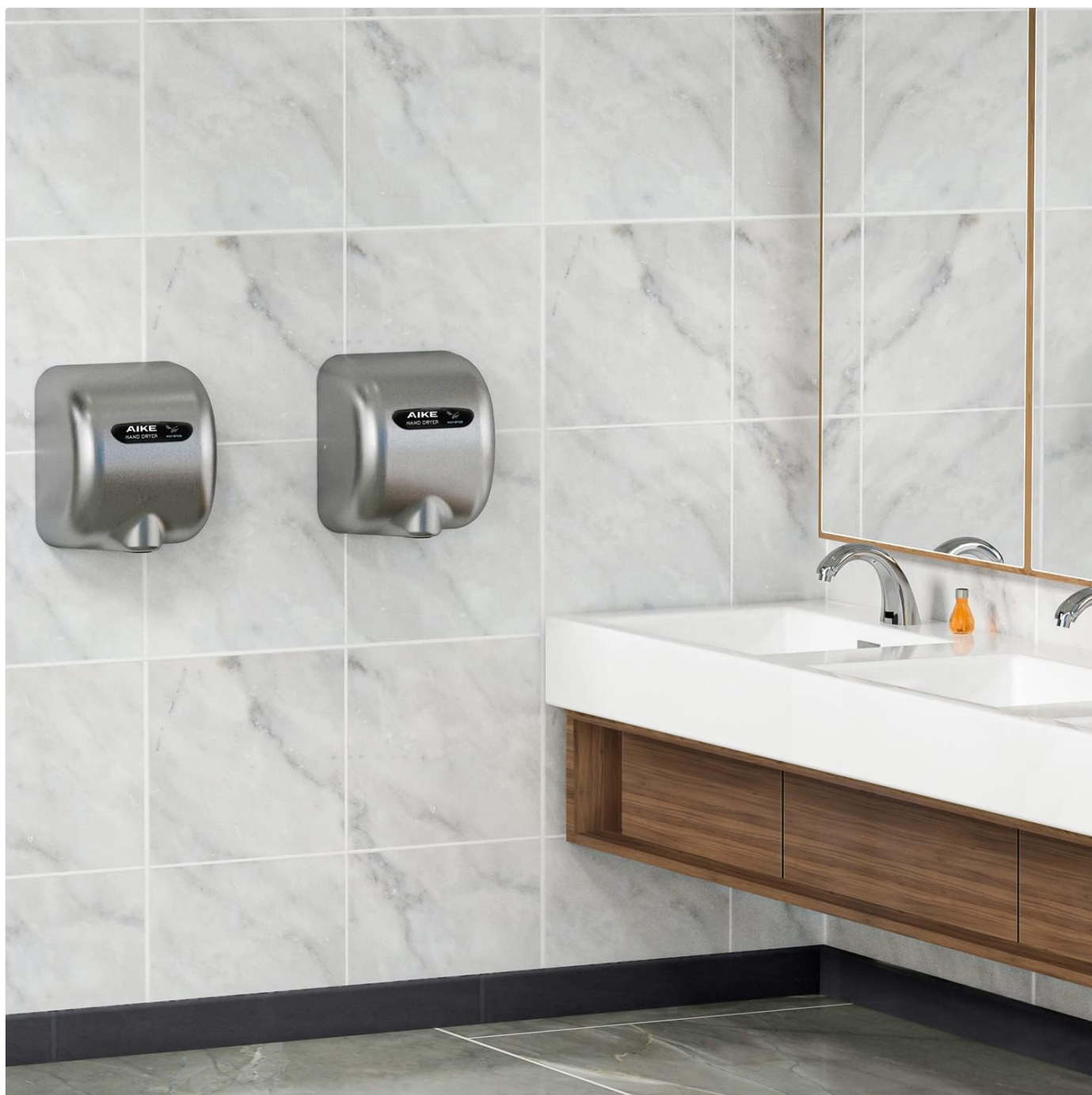
Image: Two AIKE hand dryers mounted on a tiled wall in a commercial bathroom, demonstrating typical installation in a washroom environment.
