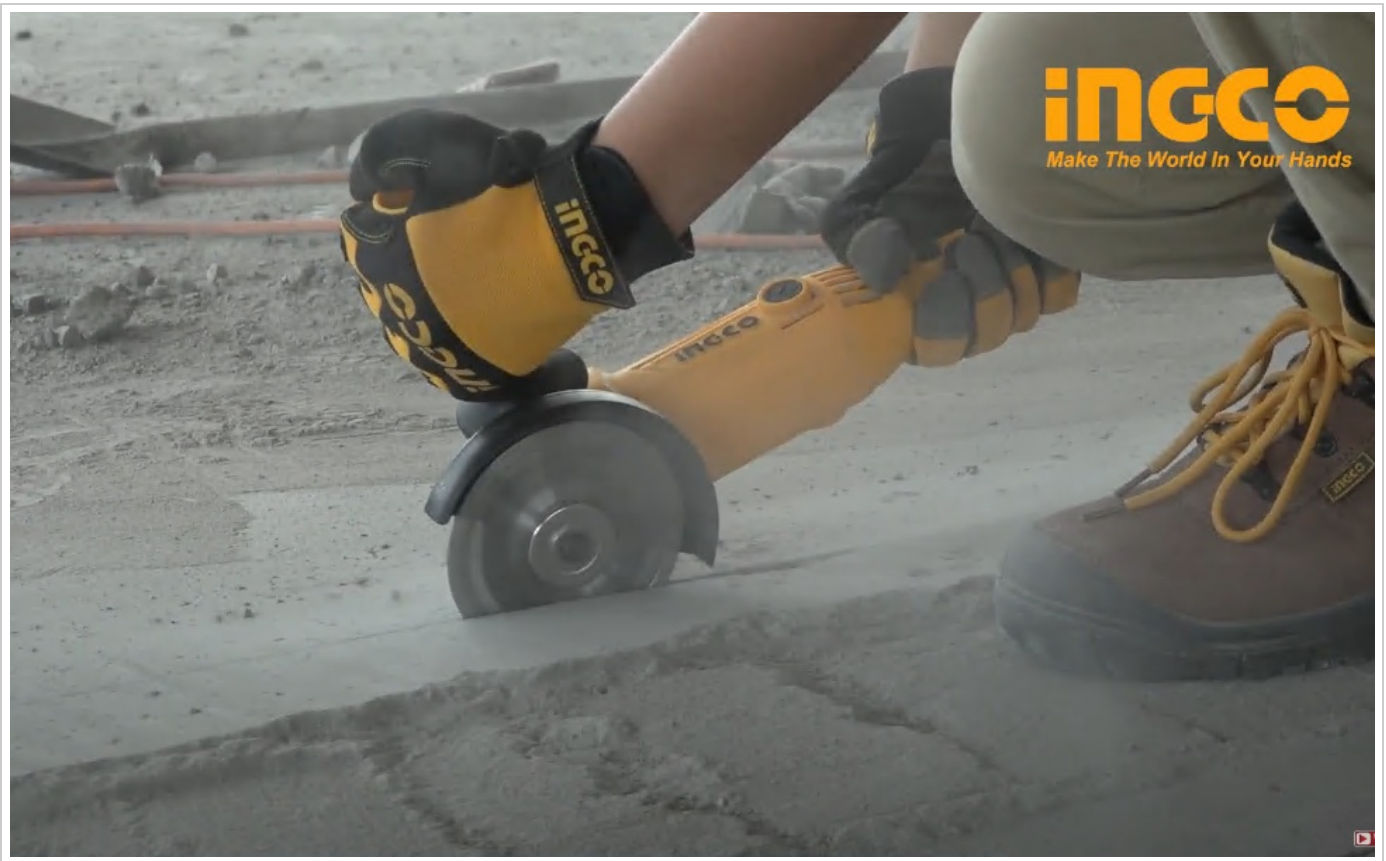
Figure 4.2: An angle grinder being used to cut concrete. This illustrates the tool's capability for heavy-duty cutting tasks on hard materials, emphasizing the need for proper technique and safety gear.
