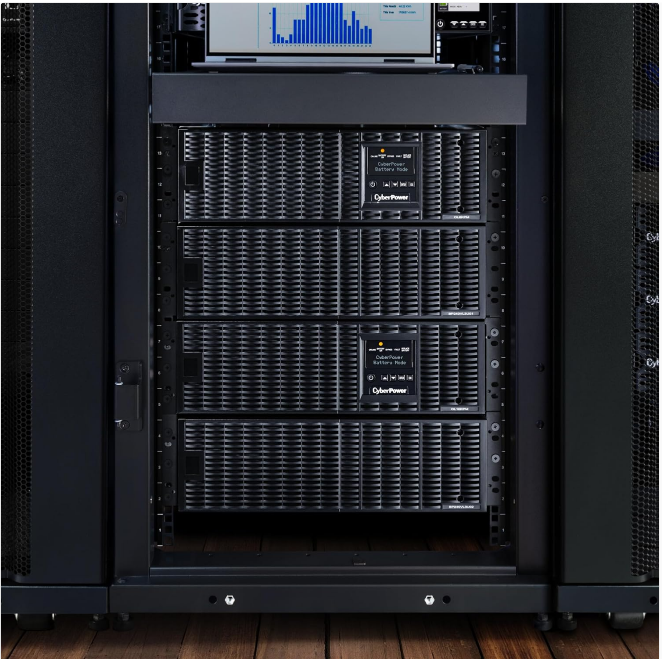
Image: Multiple CyberPower OL10KRT UPS units and their extended battery modules installed within a server rack, demonstrating a typical rackmount setup.
