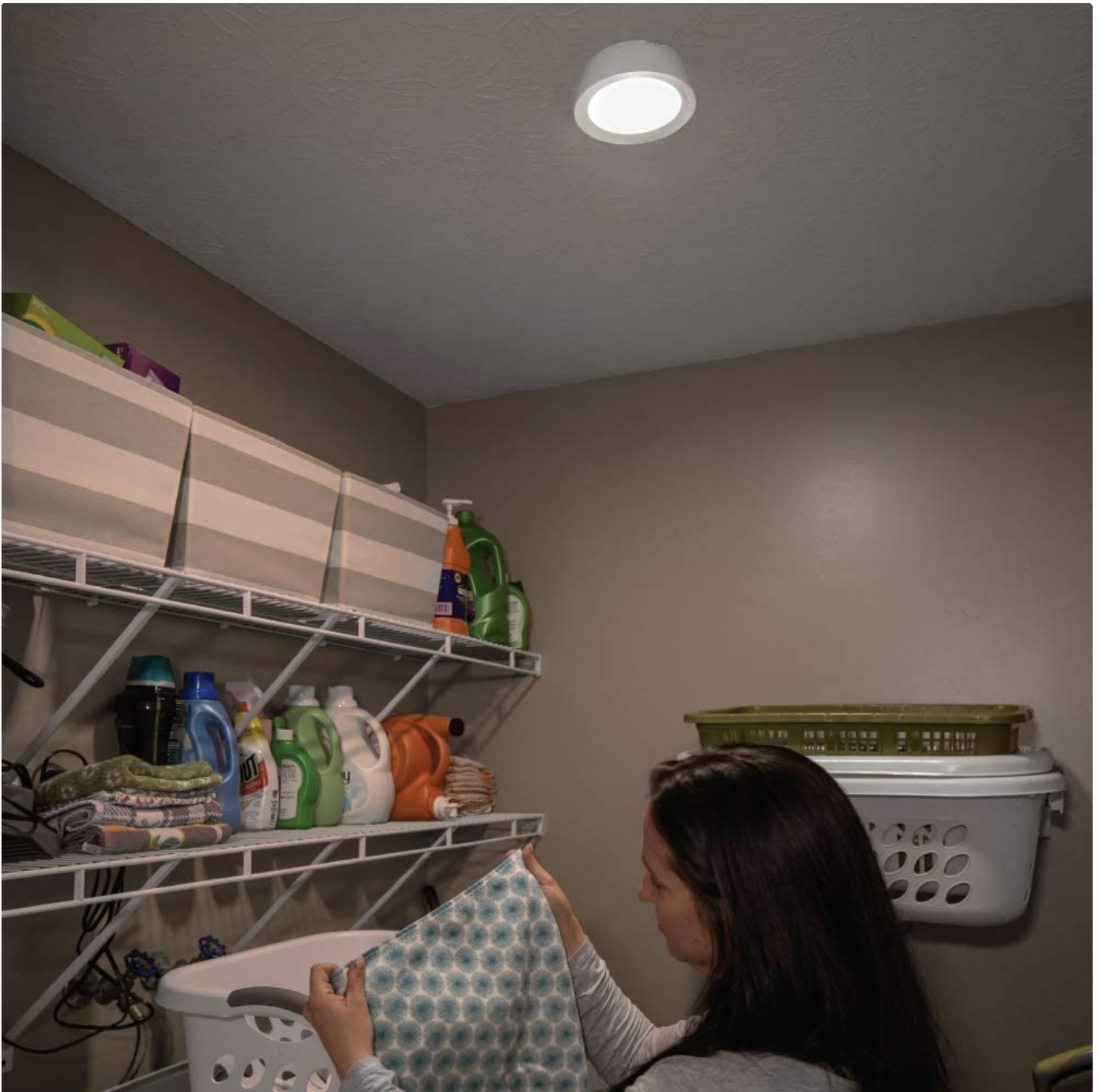
Image: The Mr Beams MB981 LED Ceiling Light installed on a ceiling, providing illumination to a laundry room with shelves and baskets.
