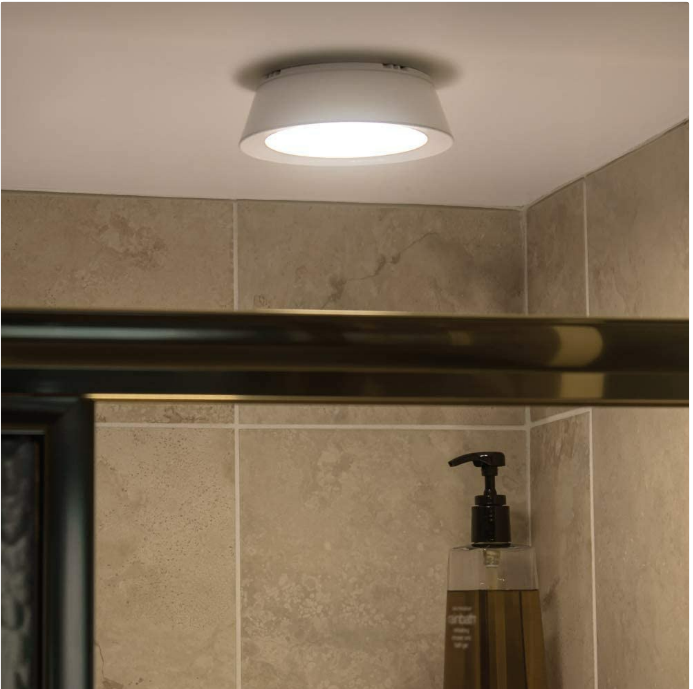
Image: The Mr Beams MB981 LED Ceiling Light installed on a shower ceiling, providing light in a tiled shower stall.
