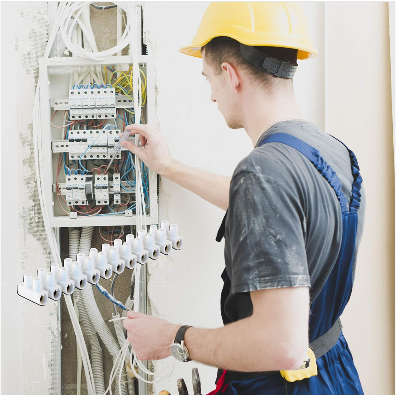
Figure 4.1: An electrician working with electrical wiring and terminal blocks. This image illustrates a typical installation environment where terminal blocks are used to organize and connect wires within an electrical panel or junction box. The professional is wearing appropriate safety gear, including a hard hat.
