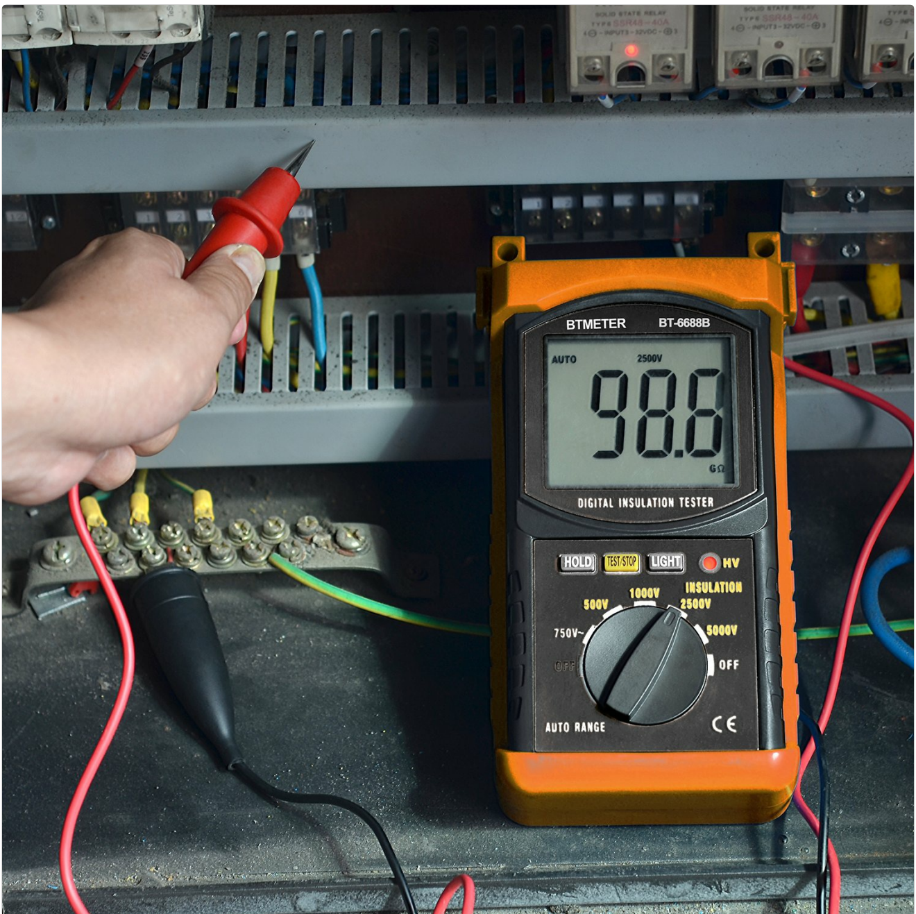
Image: The BT-6688B tester actively measuring insulation resistance on an electrical panel, demonstrating a typical application.
