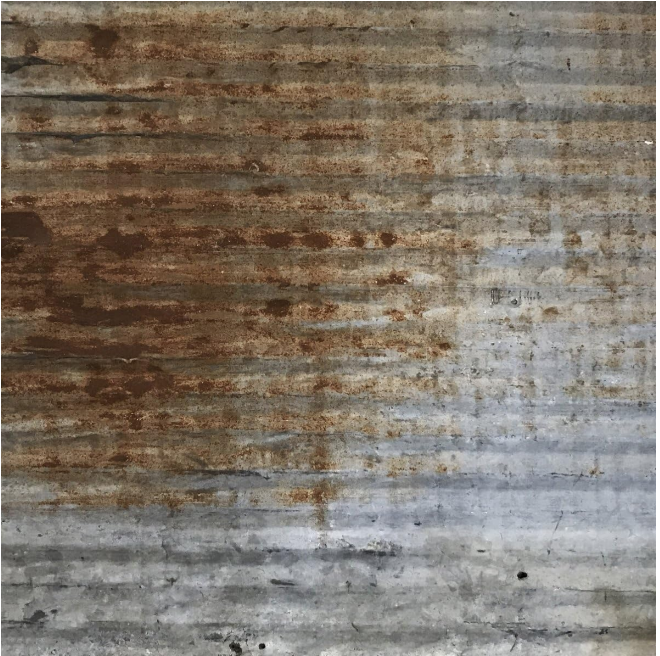
Figure 9.4: Detail of a rusted corrugated tin tile.
