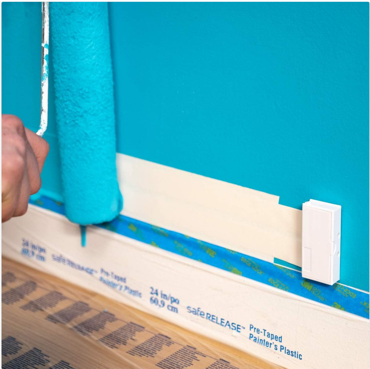
Image: Painting over the installed Ghost Wire to blend it with the wall color, showcasing its discreet design.
