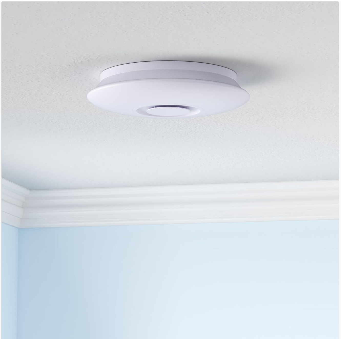
Image 5.1: HOREVO ceiling light installed.
