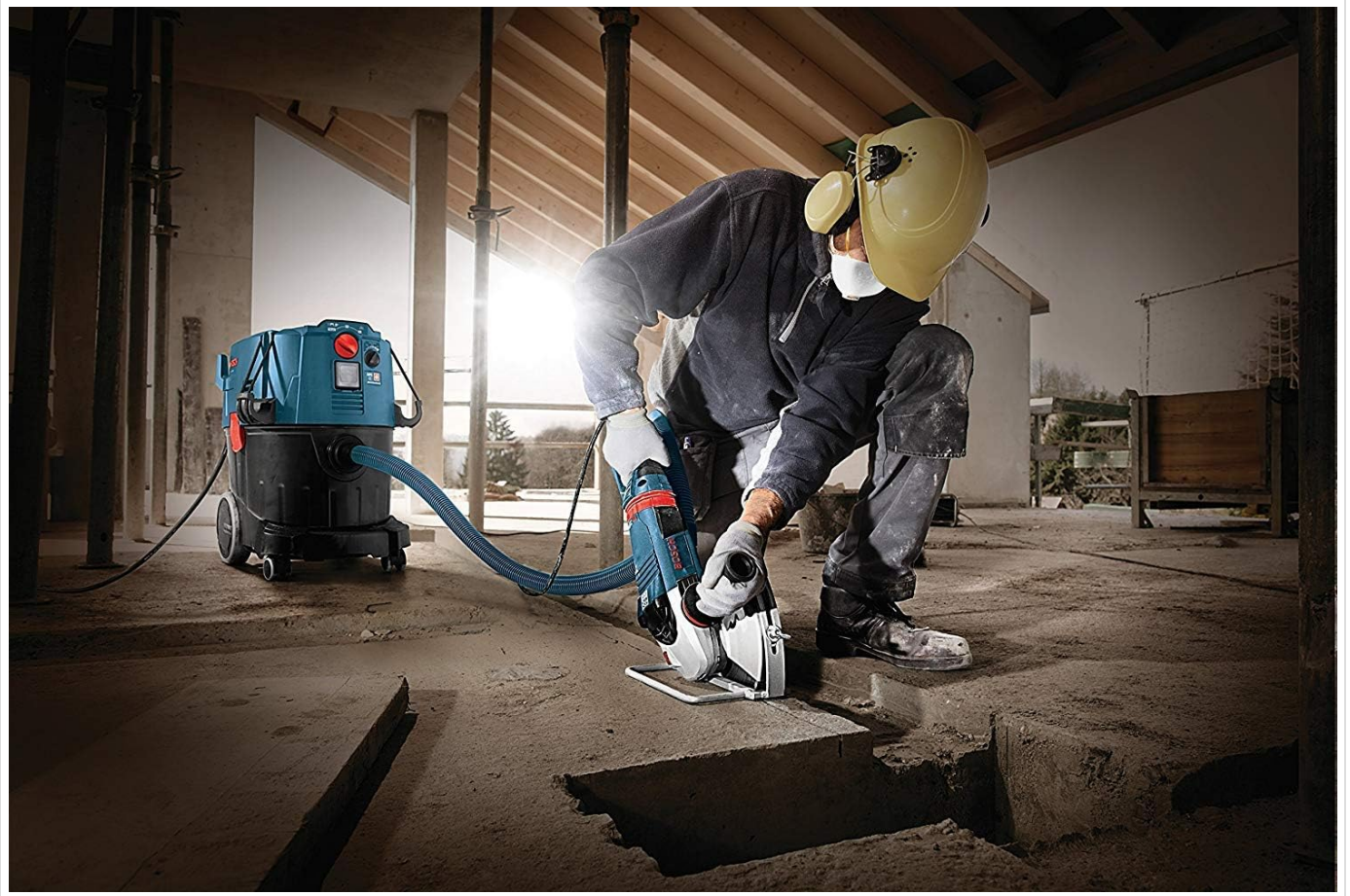
Image: A worker using the BOSCH VAC090AH dust extractor connected to a concrete grinder, demonstrating power tool activation in a construction setting.
