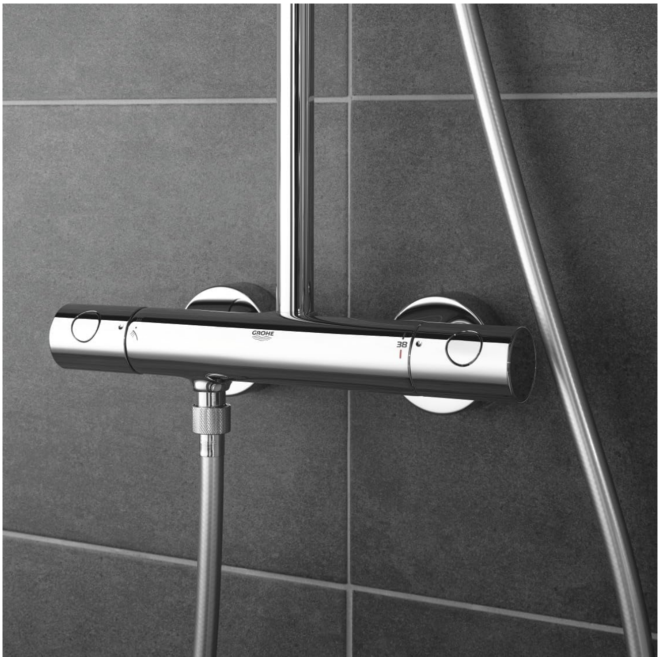
Figure 4: Close-up view of the thermostatic mixer, showing temperature and flow controls.
